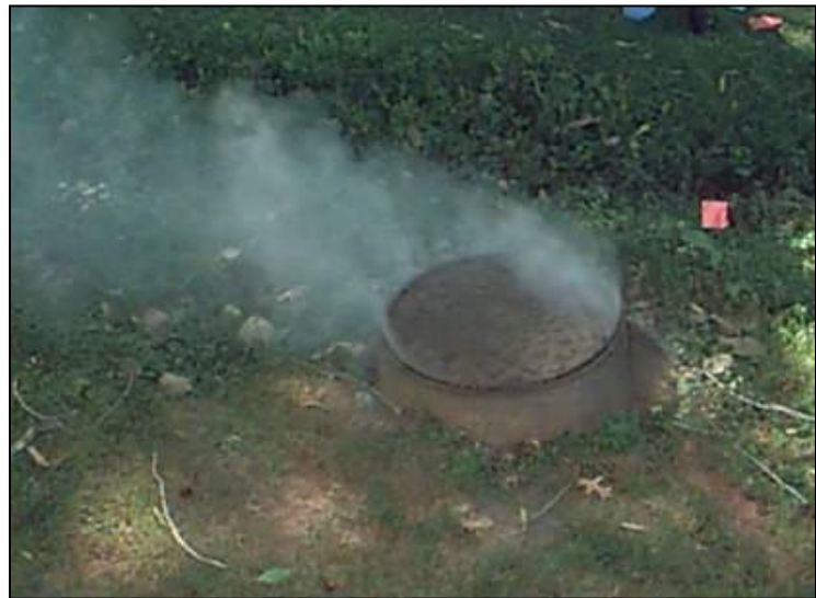
FIGURE 1.3.1 SMOKE INDICATING AN INFLOW SOURCE AT A MANHOLE
