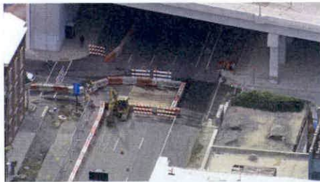
LOUISVILLE, Ky. — A sewer collapse in downtown Louisville has closed several streets.
