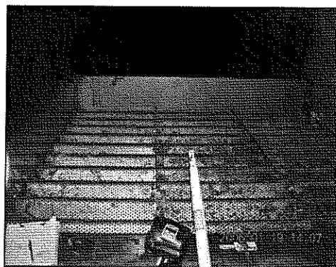
Wave Screen installed in MSD CSO area.
