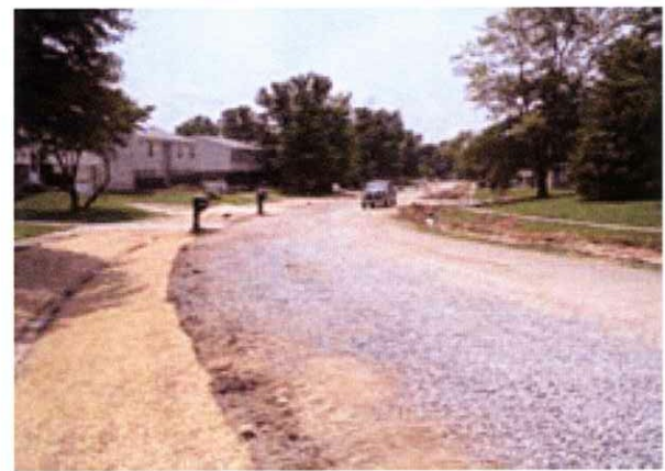
A sewer rehabilitation project along Running Fox Circle has corrected low spots in the sewer line which have caused repeated backups for 13 of 30 area properties in the past five years.
