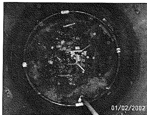
CDS Unit installed in MSD CSO area.
