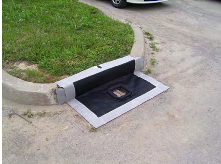
Catch Basin Silt Filter System at CMF
