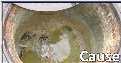
Grease Accumulating in Sewer Manhole
