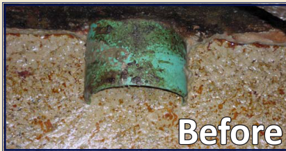
Poorly Maintained & Malfunctioning Grease Trap
